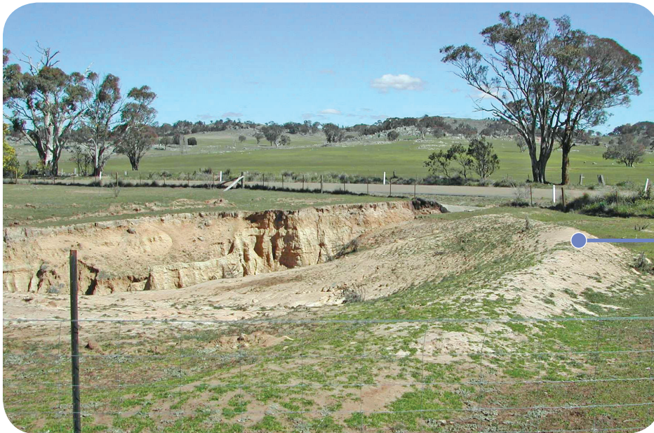
Lateral gully protected by diversion bank.
